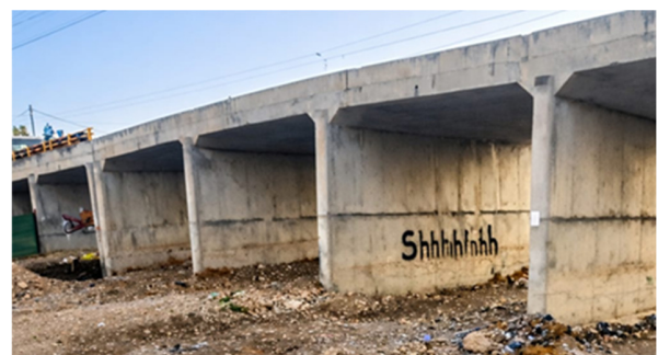
Fig. 6. Initial erosion section of the bridge.
