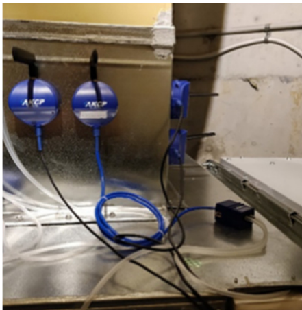
Fig. 4. Sensor installation in the air duct.
