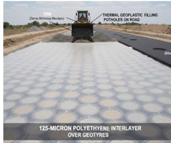
Fig. 2. Preparation of road with waste geo-tires, 125 µm polyethylene sheet as interlayer, and potholes filled up with Thermo-Geo-Plastic (TGP) material between BC.
