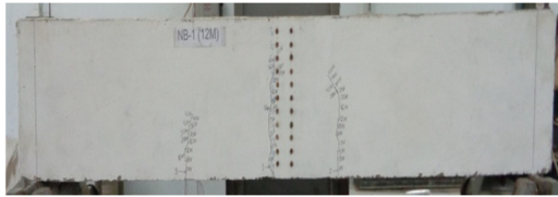
Fig. 12. Cracking of natural aggregate beam (12-month loading)
