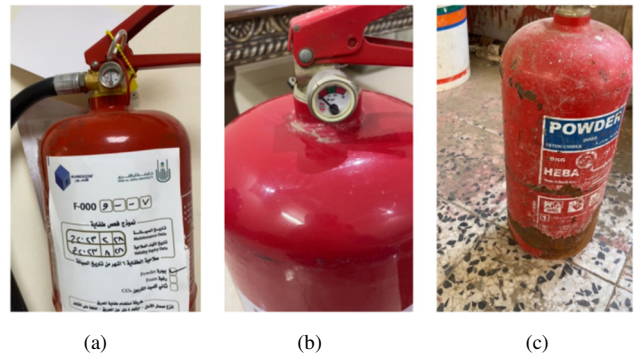
Fig. 2. Dataset examples of defective and non-defective fire extinguishers: (a) Non-defective extinguisher meeting all conditions; (b) Defective extinguisher lacking both safety pin and hose, and the gauge indicator being in the red area; (c) Defective extinguisher showing rust and absence of the hose.
