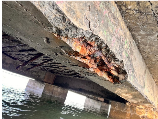
Fig. 1. Spalling of RC beams due to corrosion.
